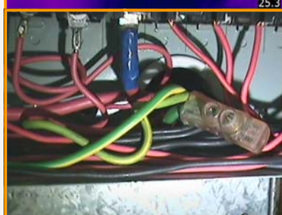
Earth wire fault.
